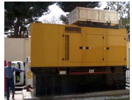
PERMIT™ Filter/Silencer Unit Installed on Diesel Back-up Generator
