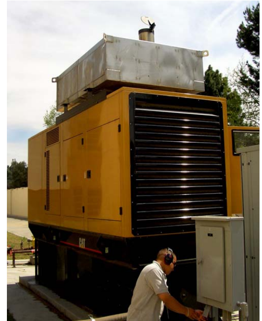
A PERMIT™ Filter/Silencer installed on an emergency generator to eliminate visible black smoke and odor. (Note stack at top of photo)
